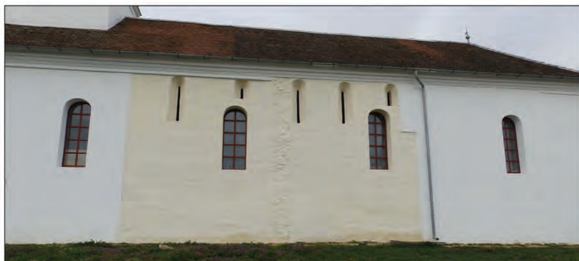
Fig. 2. Scale plan and images of the southern facade of the church, with the Romanesque wall.
